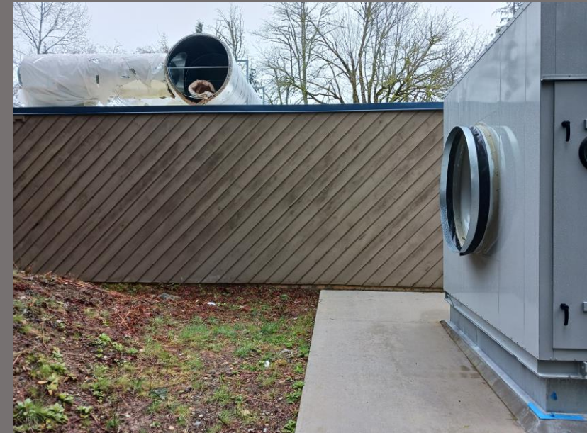
Photo: Indoor Range HVAC System Progress Photos
