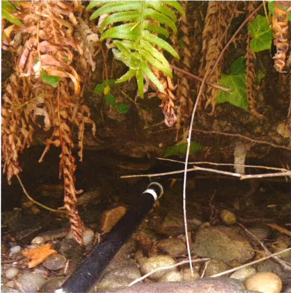
Erosion undercut along West Lake Samish Dr. Distance from tip of paddle to white tape is two feet. Photos on following two pages show how close the road edge is to the lake.
