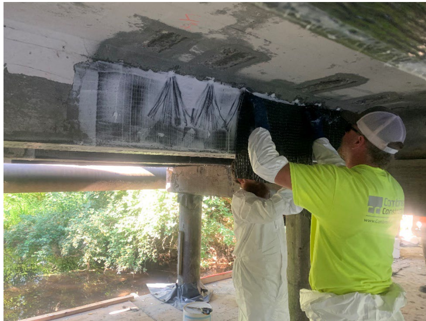
Installation of carbon fiber reinforced polymer strips to the existing girders on the Nulle Road/Friday Creek Bridge No. 106.
