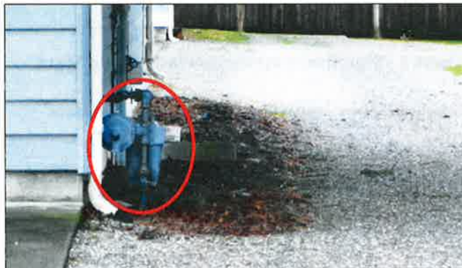
Gas infrastructure vulnerable to outside force damage.
