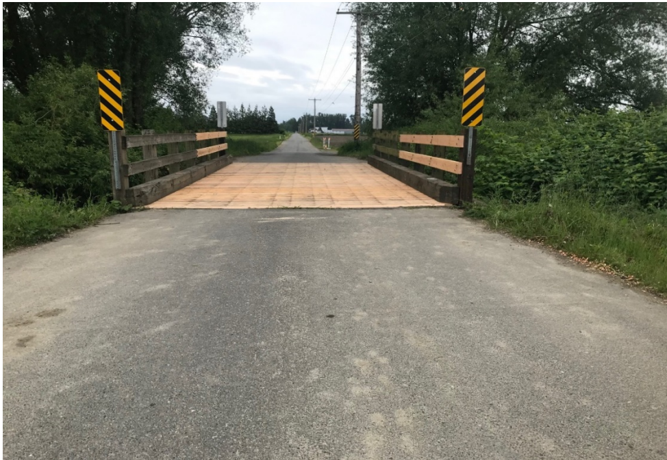
Photo of the completed repairs to the Flynn Road/Fishtrap Creek Bridge No. 51.
