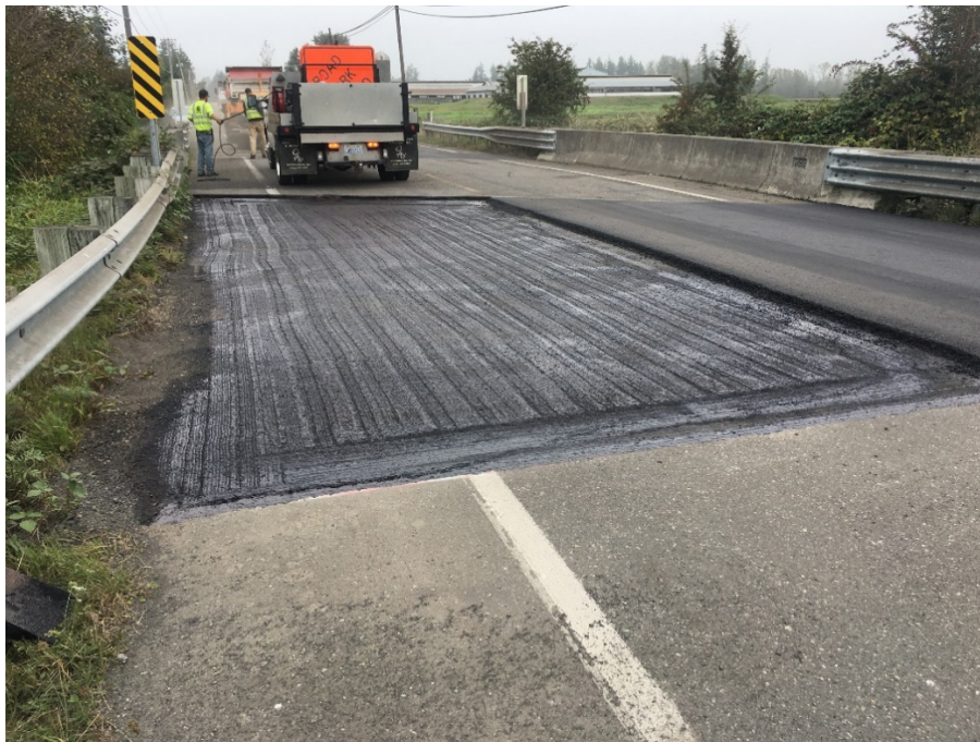
Photo of typical bridge approach repair completed as part of the 2020 Small Area Paving Project.
