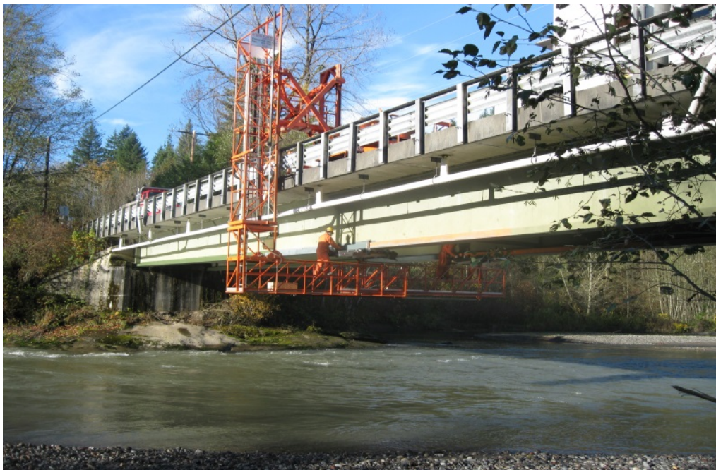
Photo of M&O's bridge inspection platform in use on Mosquito Lake Road/NF Nooksack River Bridge No. 332
