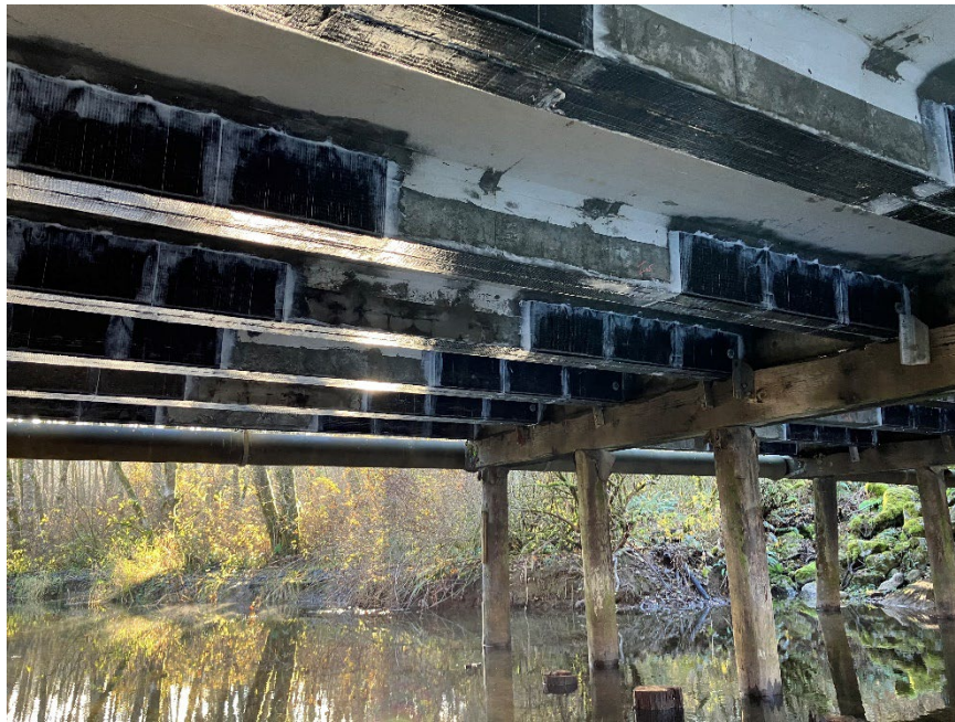
Picture of newly completed carbon fiber reinforced polymer strips to the existing girders on the Nulle Road/Friday Creek Bridge No. 106.
