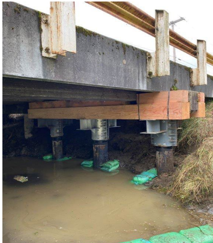
Completed helper timber cap installation at north abutment of Gillies Road/Sumas River Bridge No. 309
