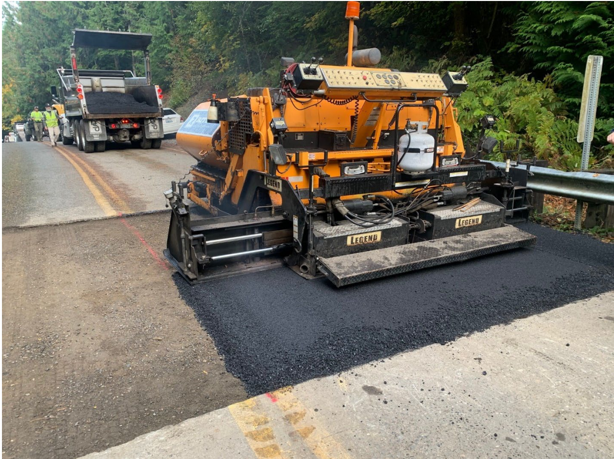
Photo of typical bridge approach repair completed as part of the 2021 Small Area Paving Project.
