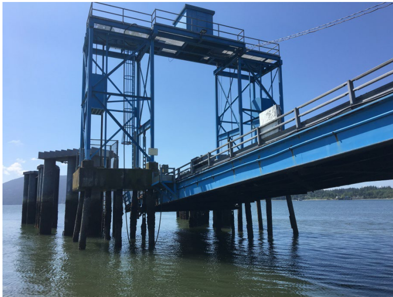
Gooseberry Point Terminal
