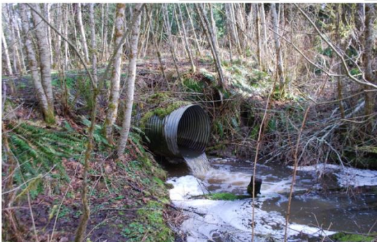
No migration – fish stuck below the culvert
