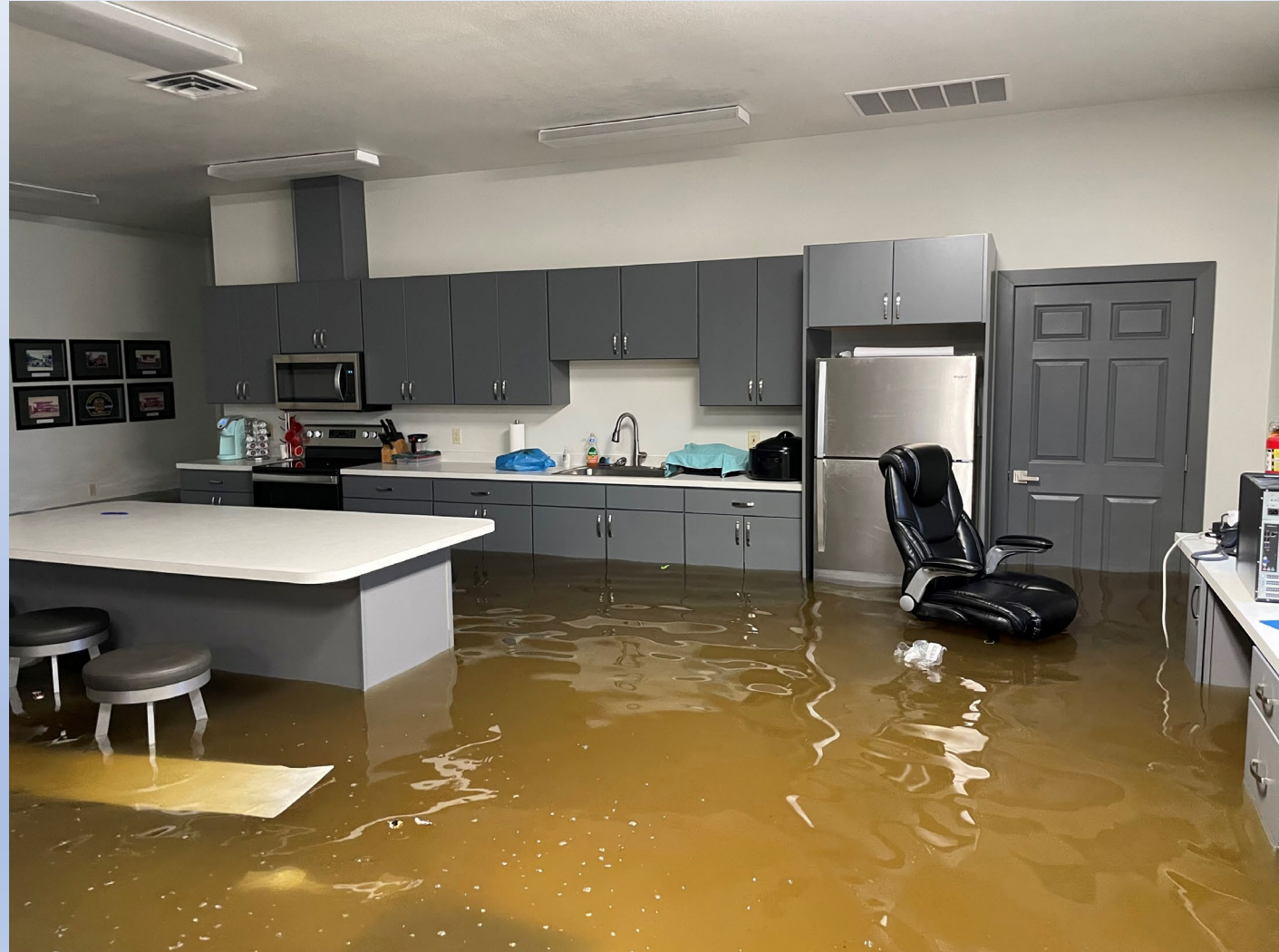
Photo: Inside Whatcom County Fire District 17 Station, Sandy Point -King Tide Event, 2022
