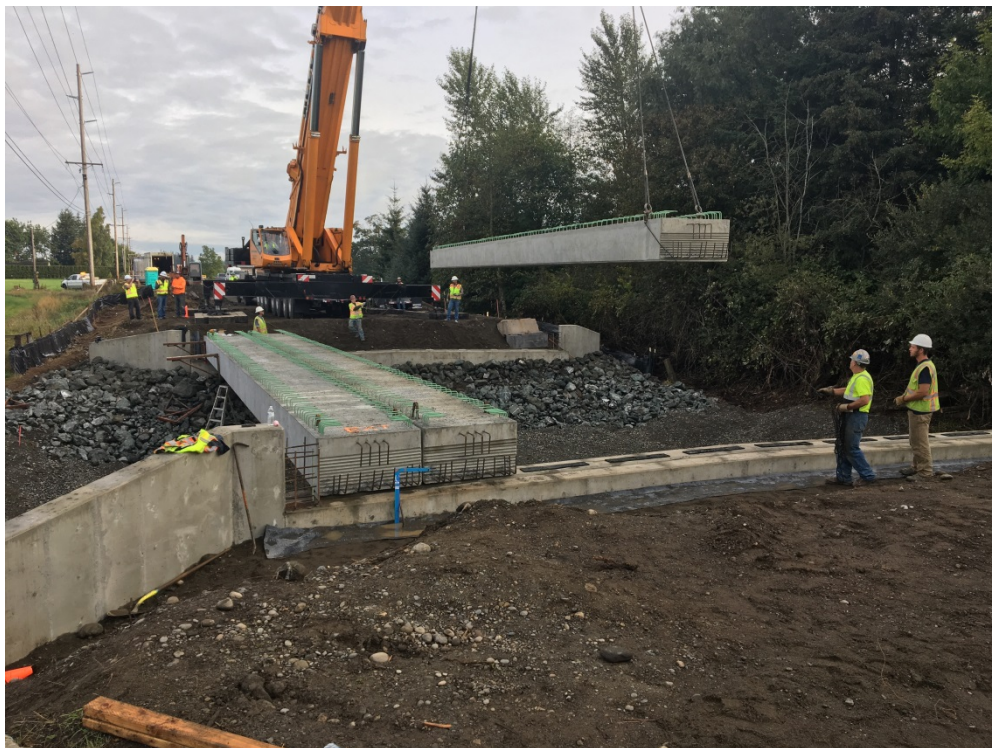
Setting girders during construction of the new Hannegan Road/Ten Mile Creek Bridge No. 236
