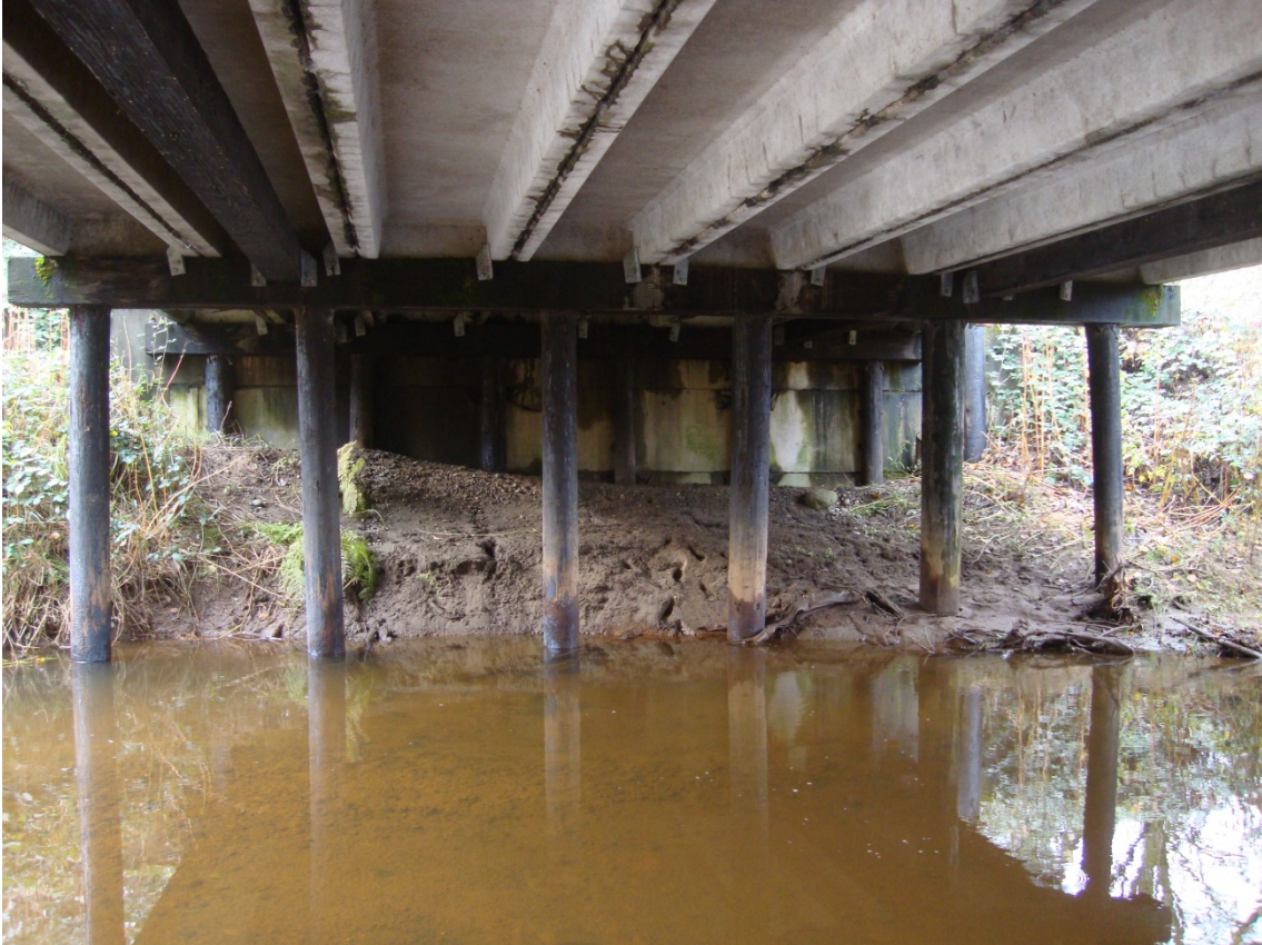
W. Badger Road/Bertrand Creek Bridge No. 50 is typical of our channel beam girders supported by timber piles and caps
