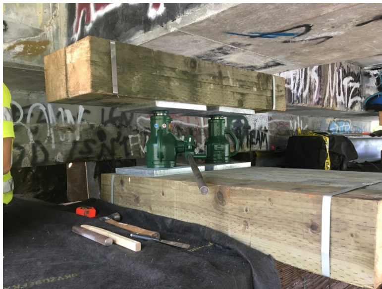
Photo of wood cribbing and jacks used for temporary shoring during construction
