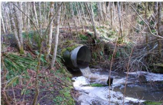
No migration – fish stuck below the culvert
